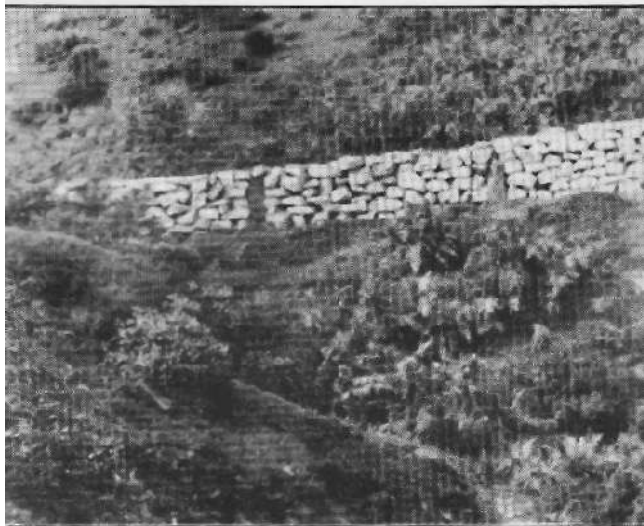
COUMS. ILLUSTRATING SINKING OF ROAD.
